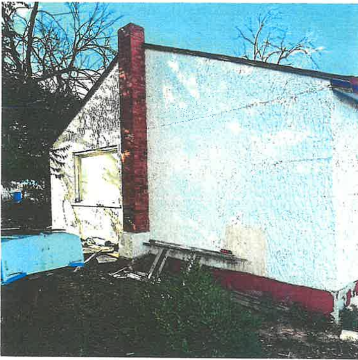
View Northwest from SE view of garage. Area shown is where proposed shed will be mounted against back wall of garage.
